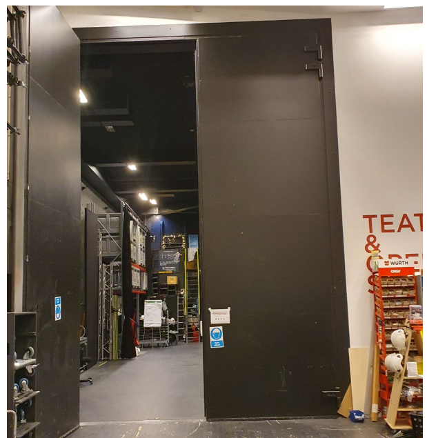
Stage Fire Door
