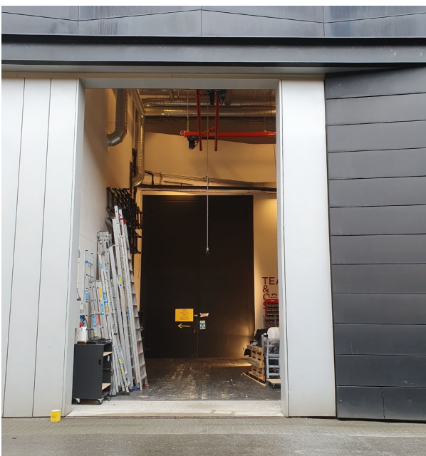
Loading Bay Door
